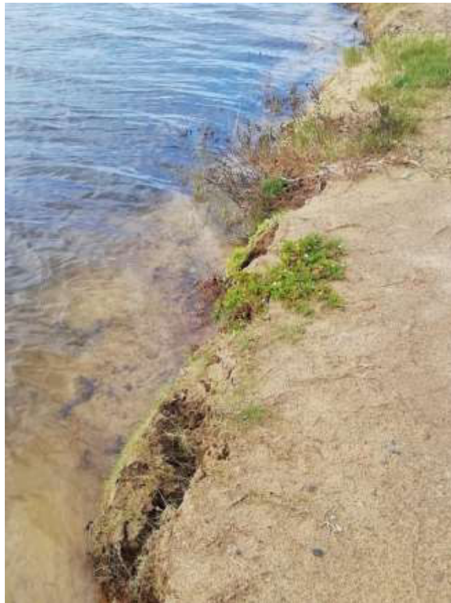
Riet River Embankment Erosion
